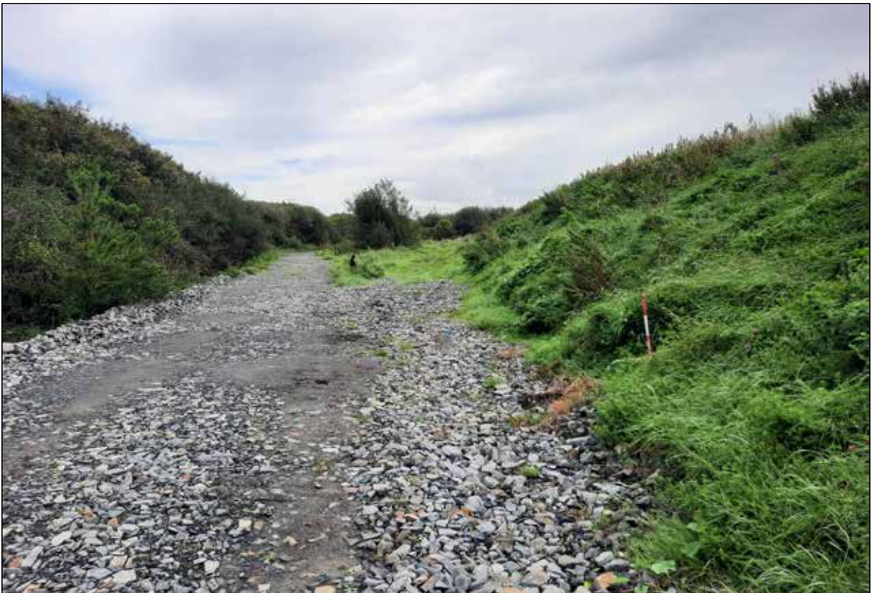
Plate 12 - View of northern boundary of development from CH027 to CH028, facing NE
