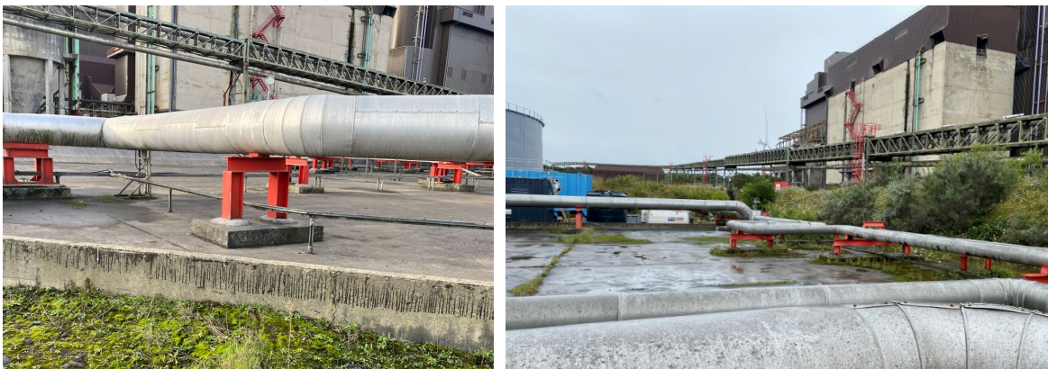
Figure 2.2 Existing floors to the south of the storage tanks in each HFO bund
